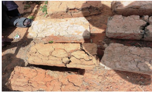
Figure 15. Cracks propagation due to high clay content
